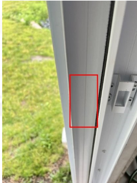
There should be a catch to latch the door in the closed position.
