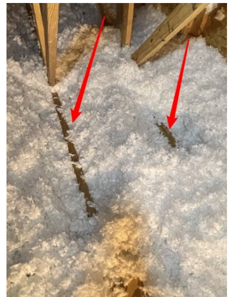
Exposed top cords are at 5 1/2 inches. There is not enough insulation in the attic to cover them with 6 additional inches.
