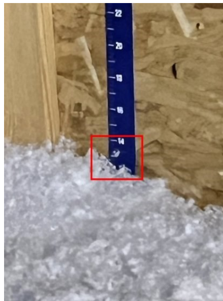
2 1/2 inches short at insulation marker
