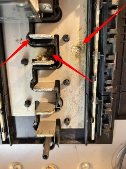
Damaged electrical panel
