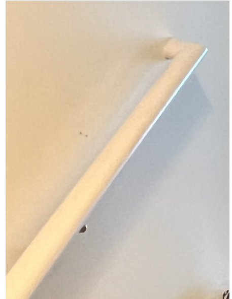
No support near the top of the railing.
