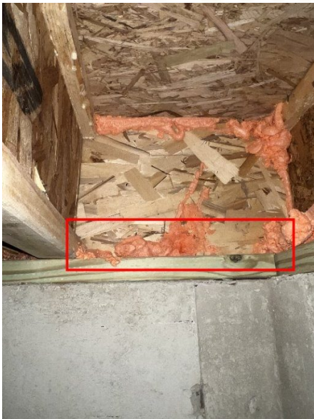
front right corner no bolt
