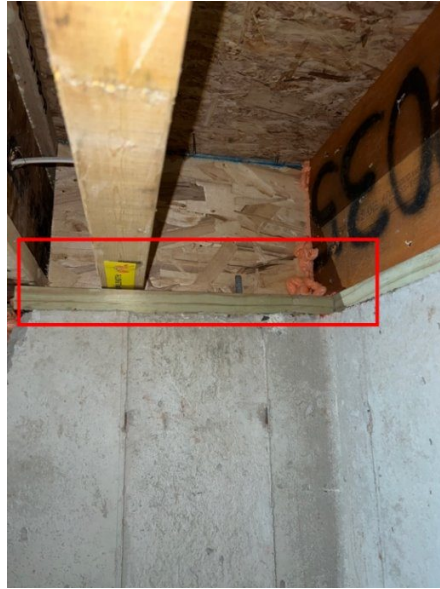
only one bolt on this section
