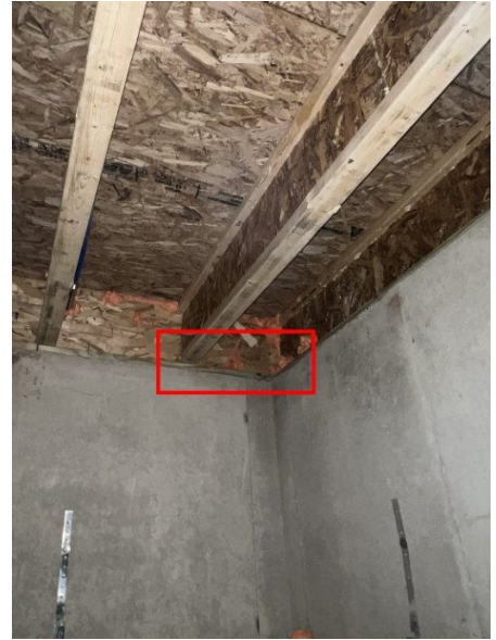
front right corner no bolt
