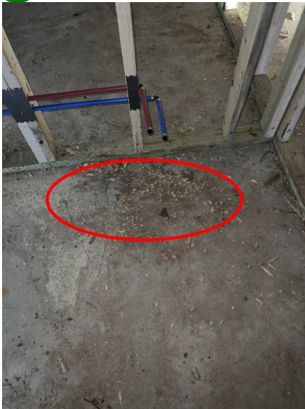
no drainpipe for bathroom sink
