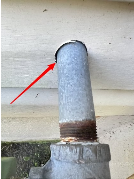
Gas line left side of house
