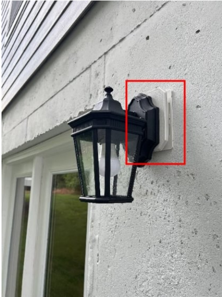
Incorrect siding block application
