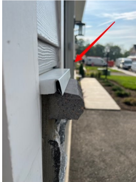
coping flashing sloped the wrong way.
