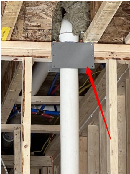
Steel plate not adequate
