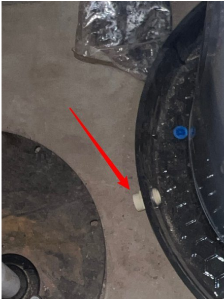
drain line needs to be installed and extended to the sump
