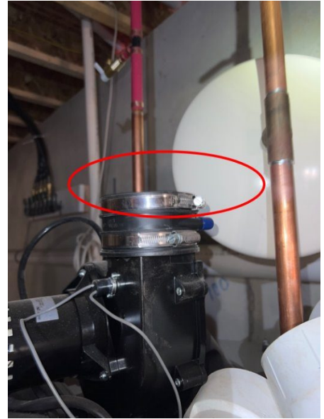
flue pipe needs to be connected
