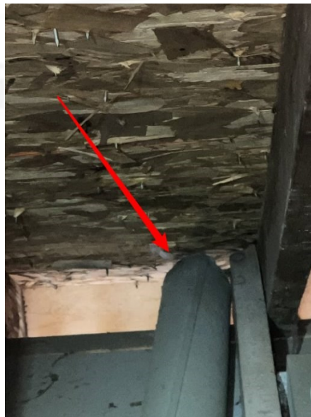
venting into the soffit does not work
