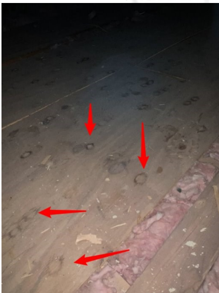
water stains from condensation dripping off of the nail ends
