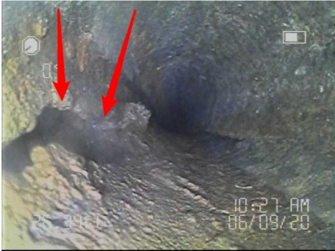
Crack in sewer line 25 ft. from basement clean out.
